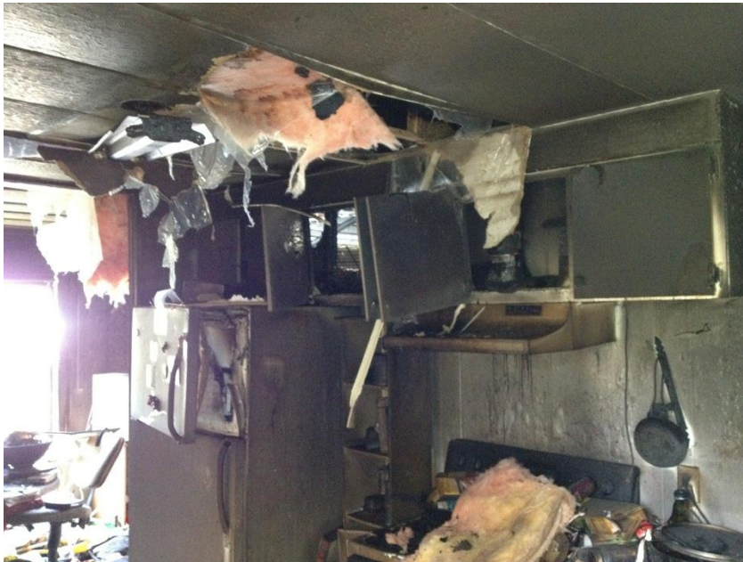
Damage from fire at local residence.
